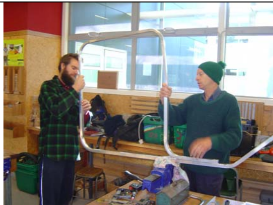
Telescoping the two halves of the frame to get the right width for the bins.
